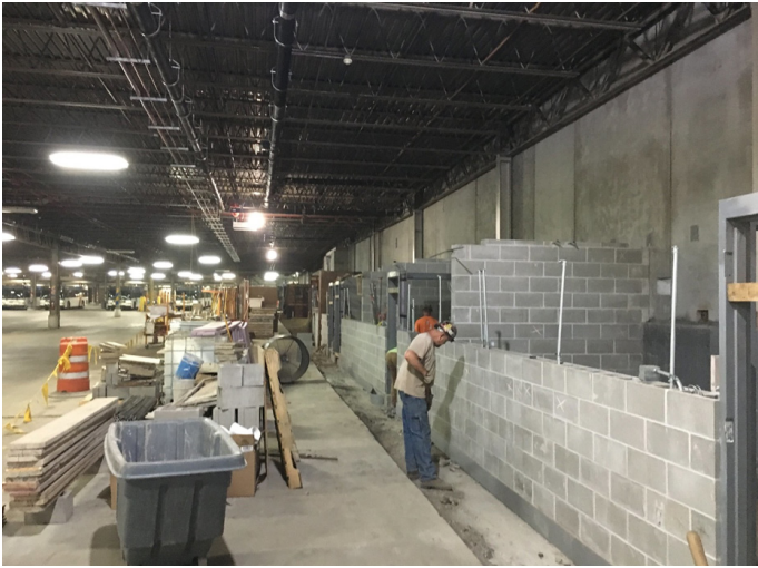
1101 East Washington Ave. Phase 1 – Service Lane Addition, City of Madison Flickr (September 19, 2019)
